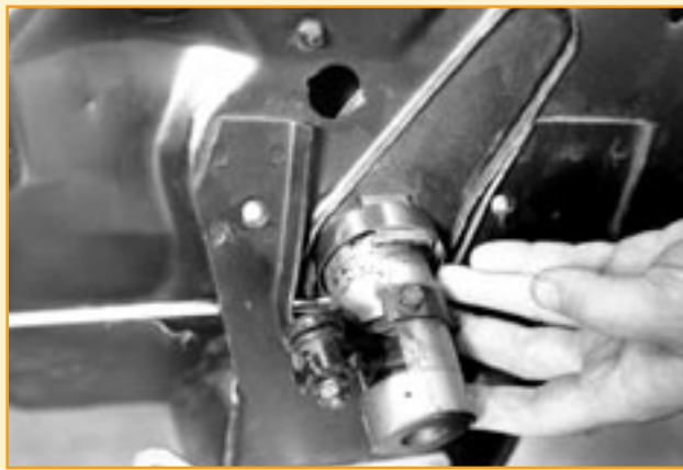
The new bracket bolts to the firewall from inside the passenger compartment. A clamp secures the tab of the bracket to the steering column itself.
