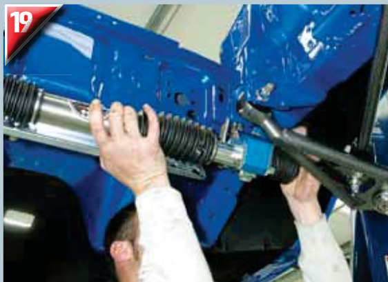
19 Richard mounts the rack, starting each of the Allen-head bolts, then checks position.
