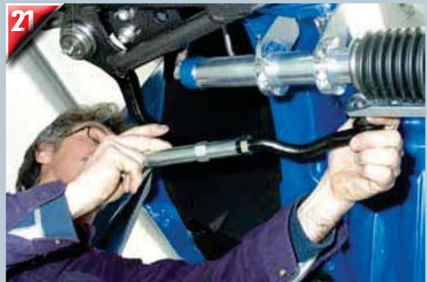
21 Terry Simpson of The Restomod Shop installs tie-rod ends and the TCP bumpsteer kit. TCP provides two attachment points for inner tie-rod ends. For '65-'66 Mustangs, it attaches to the outermost hole on the steering rack. For '67-'70, use the innermost hole because the steering rack is wider.
