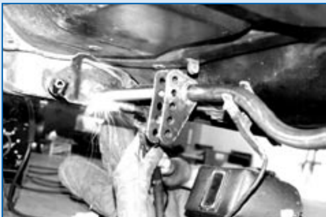
With the rear brackets tacked in place, and after making sure everything is straight and square, the front crossmember is tacked to the frame. The ladder bars are then removed from the front brackets, and the crossmember is welded to the frame.
