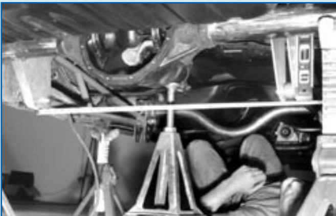
Constant use of a tape measure is critical to ensure the success of any chassis or suspension installation. Here, the distance between the brackets is verified after they are tacked to the housing.
