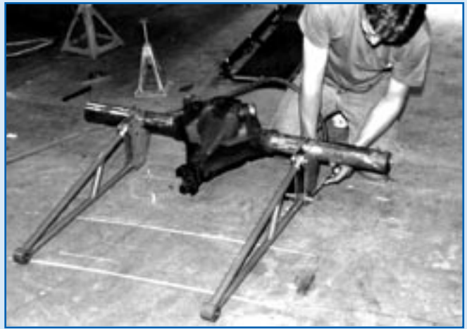
The housing is brought back out from under the car and the ladder bars are removed from the brackets. The ears at the top of the housing, used for mounting the stock link bars, will be removed to provide clearance for the panhard bar.
