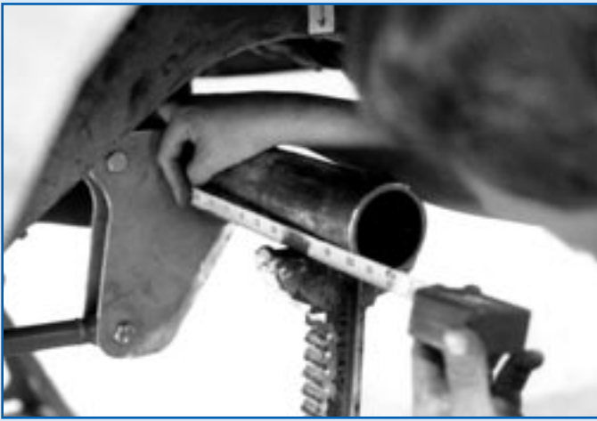
Bumping the brackets into the housing will undoubtedly jostle it around; all measurements must be rechecked before firing up the welder.
